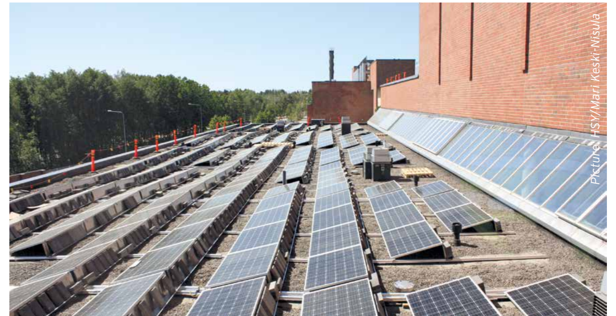
Solar panels were installed on the roofs of Viikinmäki wastewater treatment plant in summer 2016.
